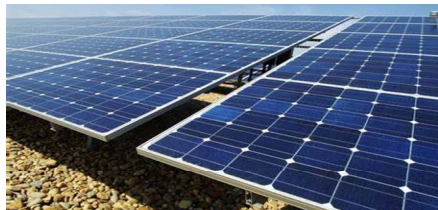
Solar Photovoltaic (PV) Array
