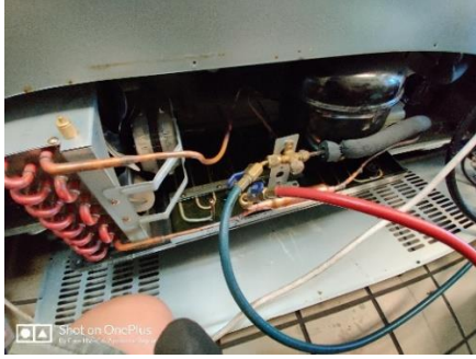
Brazed Components - Air Conditioning System
